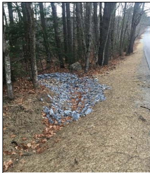
New ditch and turnout installed as part of Parker Pond Protection Project Phase II
