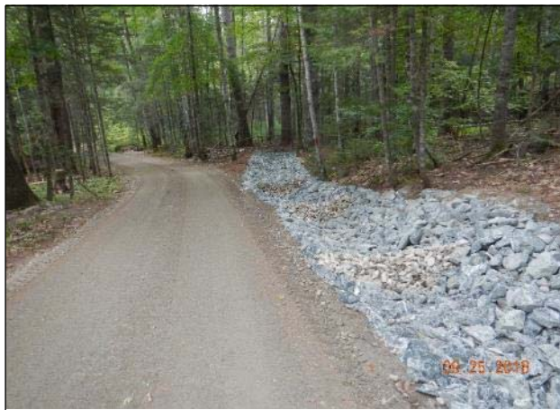
Dinsmore Road – Chronically eroding road was stabilized with crushed gravel and graded to direct runoff into rock-lined ditch and turnout.
