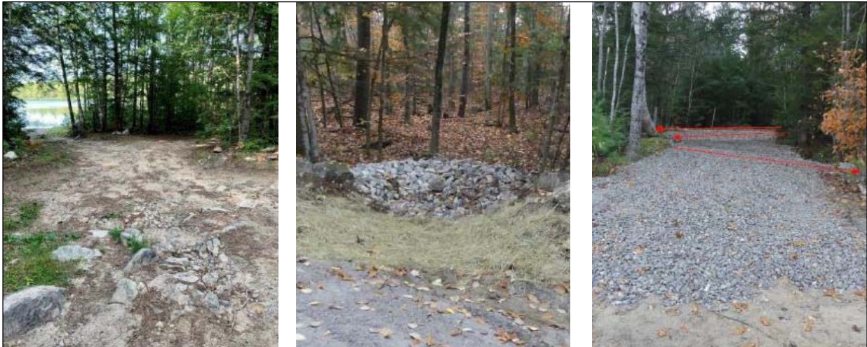
Otter Pond Lake Phosphorus Compensation Project - Lakes Environmental Association used compensation funds to address a chronic erosion problem on Otter Pond Road. Before (above left) - 1000 feet of severely eroding road directed runoff into Otter Pond. After (above middle and right) - The road was re-graded with crushed gravel, and waterbars, turnouts and level lip spreaders were installed to divert runoff into vegetation.
