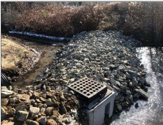
A new outlet control structure was installed for the farm's instream irrigation pond, which allows one branch of Trout Brook to freely flow downstream to improve stream oxygen and habitat.
