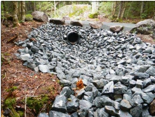
Dinsmore Road – Undersized 12” culvert was replaced with a 24” culvert and stable plunge pool.
