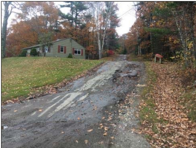
Pine Woods Road Before - Severely eroding, steep road with no stormwater controls
