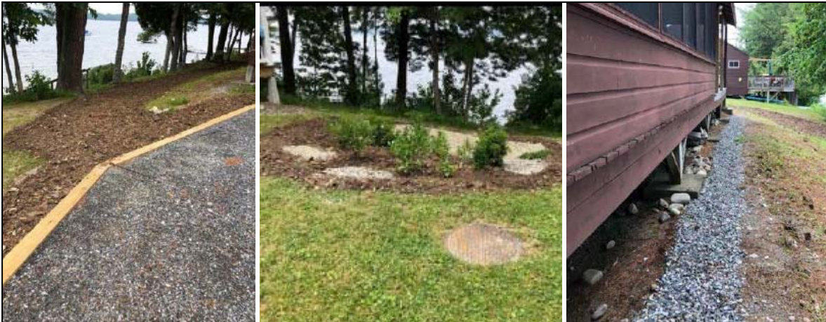
The 7 Lakes YCC installed 15 BMPs at Pine Tree Camp, including rain gardens, bluestone gravel parking areas, Erosion Control Mix on paths, cabin dripline trenches and dry wells, infiltration steps, and riprap.
